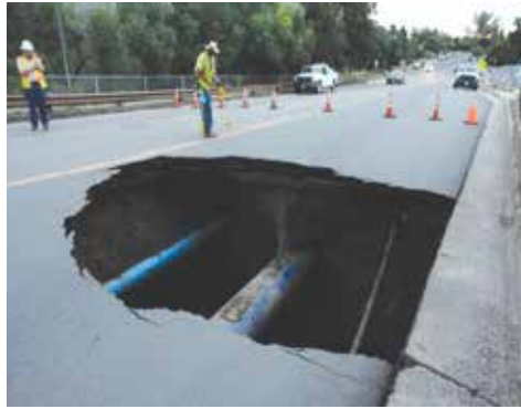
Chestnut Street Bridge sinkhole
