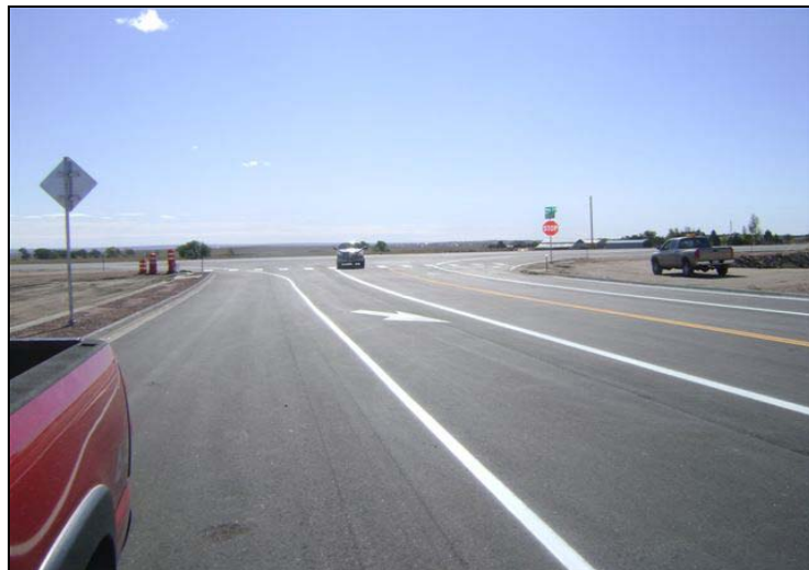
Stapleton Road (West): completed paving and striping at its intersection with US-24
