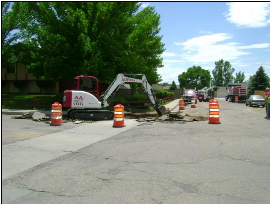
Removing Curb & Gutter and Sidewalk to Install Pedestrian Ramp at Grand Valley Dr & Silverdale Dr
